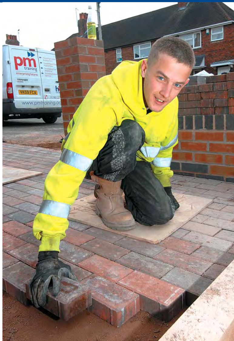
PM Training Homeworks apprentice Stefan Farr hard at work on the facelift, which has improved quality of life in Knutton.
