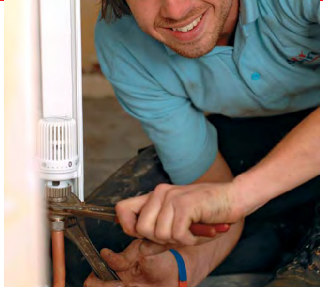
Gas engineer and plumber Rob Griffiths, hard at work in a customer's home.
